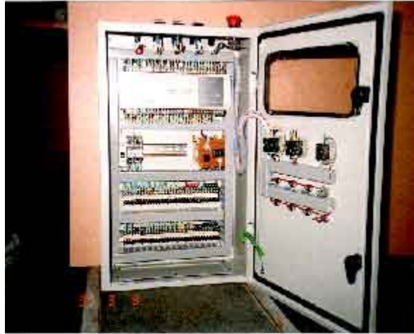
Figure 2: Typical PLC Control Panel
