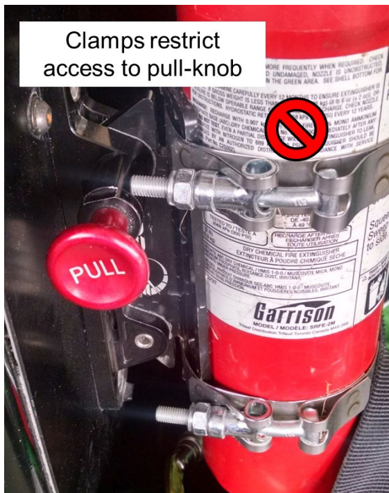
Figure B-51: Incorrect orientation of extinguisher clamps.
