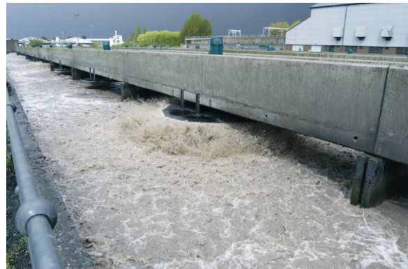
Figure 3.4 Surface aeration in activated sludge treatment plants creates aerosols which contain high amount of microorganisms. This poses a health risk to treatment plant employees and in some cases to neighbors (photo: D. Brdjanovic)
