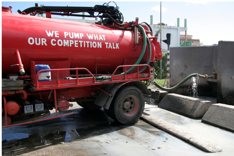
Figure 3.5 Truck discharges content of septic tanks from households to a storage tank at wastewater treatment plant Illidge Road at St. Maarten, N.A. (photo: D. Brdjanovic)
