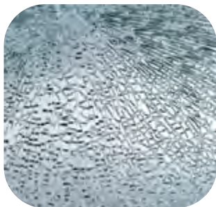
Figure 5.1. Typical fragmentation pattern of toughened glass.
