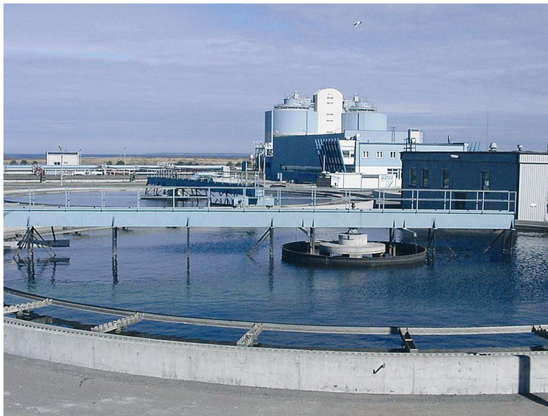
A detail of a modern treatment plant designed to remove organic matter (COD), nitrogen (N) and phosphorus (P) from wastewater of the city of Tallin in Estonia (photo: D. Brdjanovic)
